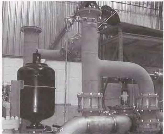
Figure 7. API 614 lube-oil console featuring 80 gallons, 500 psi accumulator; Console flow rate: 1175 gpm. Industry application: power generation.
